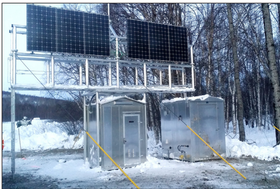
Wayside equipment at Curry is housed in new shelters and powered by solar energy generation and solid oxide fuel cell technology.
